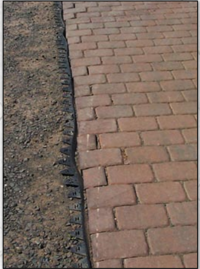
Edge restraint failure from improper product use. Flexible was used where rigid should have been used.
