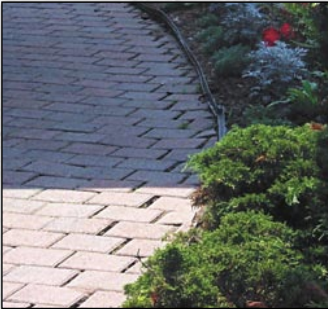
Pavement unzipping due to edge restraint failure.
